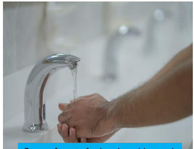
Sensor faucets for hand washing and toilets.
