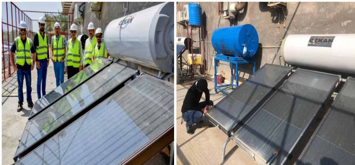
Figure 2. Solar evacuated tube collector
